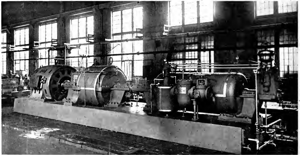
FIG. 1.—GENERAL VIEW OF 1,250-KW TURBO-GENERATOR.
